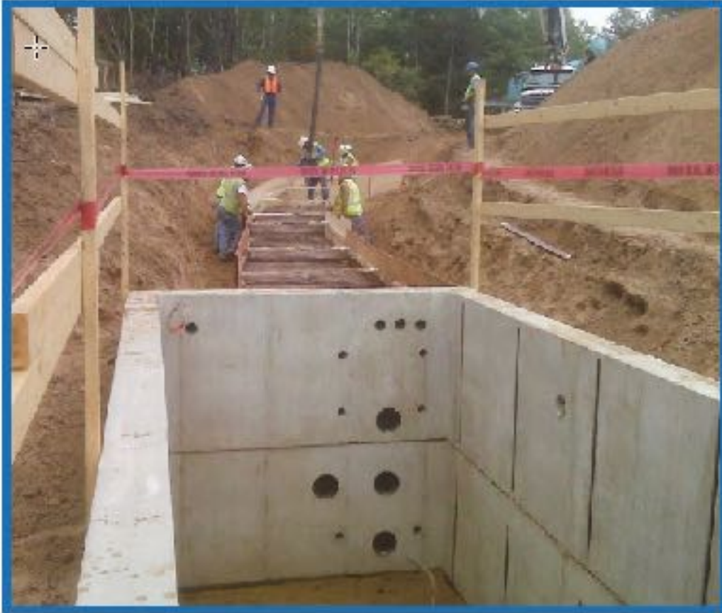
Concrete access vault for transmission line
